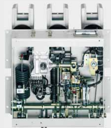
Open operating mechanism box
